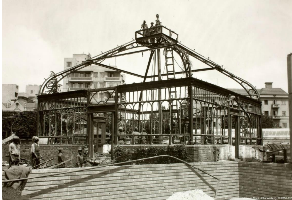
Building of the Conservatory in Joubert Park. Image courtesy Museum Africa archives.
